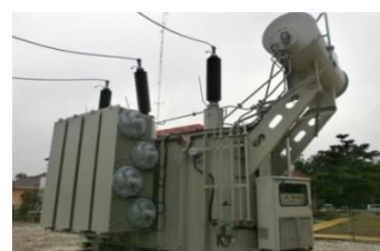
Gambar 3.2 Transformator Distribusi GI.Garuda Sakti
