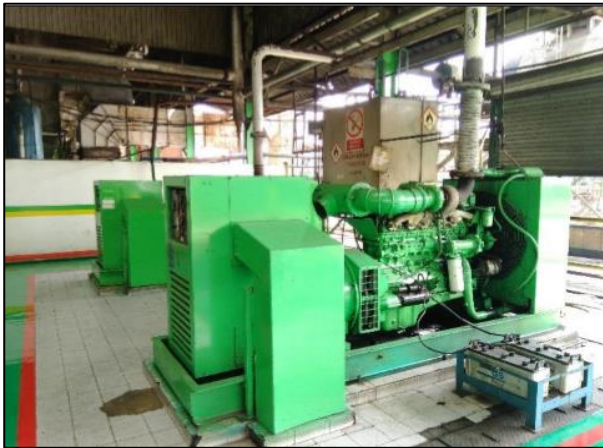
Gambar 5. Genset ( Generator Set ) (Zikir Akbar K, 2020)
