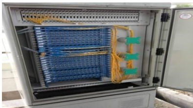
Gambar 4. Optical Distribution Cabinet
